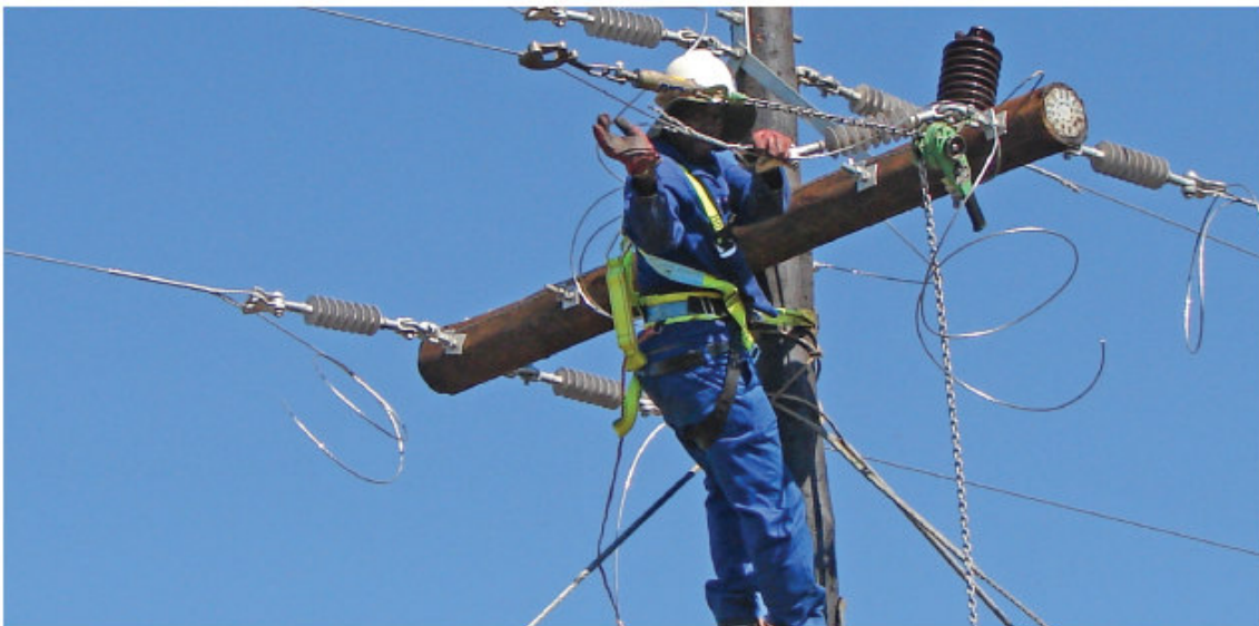
An Eskom worker connects a new line as part of an electrification project
