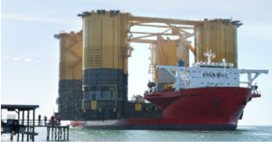
↑ The hull of the new platform for the Mars B project being moved to the Gulf of Mexico, USA.
