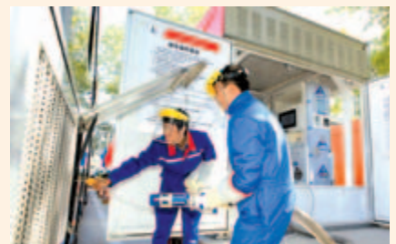
Sinopec Corp. LNG bus refueling stations were put into operation in Beijing.
