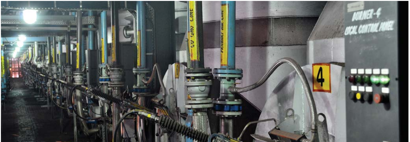
Energy efficient burners at the Indurating Machine of the Pellet Plant run on by-product gases from the Blast Furnace, CO Gas and Coal Tar
