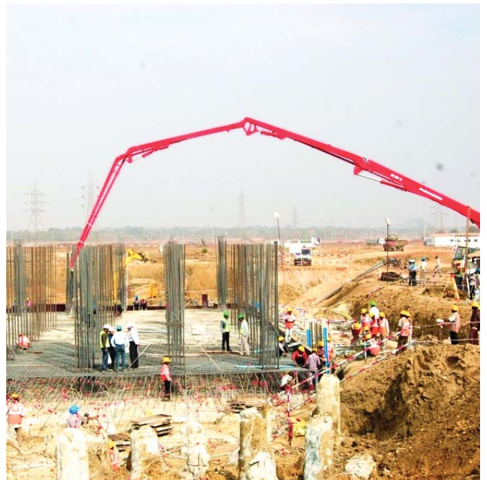
Pouring of concrete commences at the site of the Coke Oven Plant for the Odisha Project
