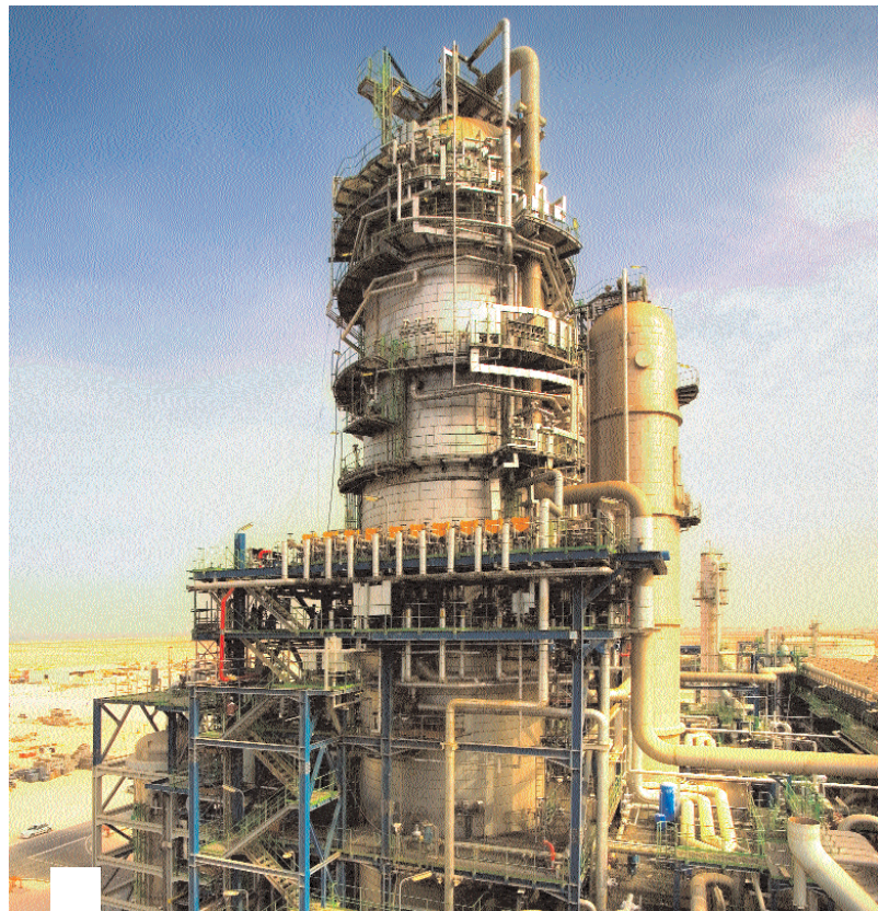
Our first international GTL venture, the ORYX GTL plant in Qatar, is nearing completion. It will start supplying high-quality GTL diesel and GTL naphtha to the world market in 2007.
