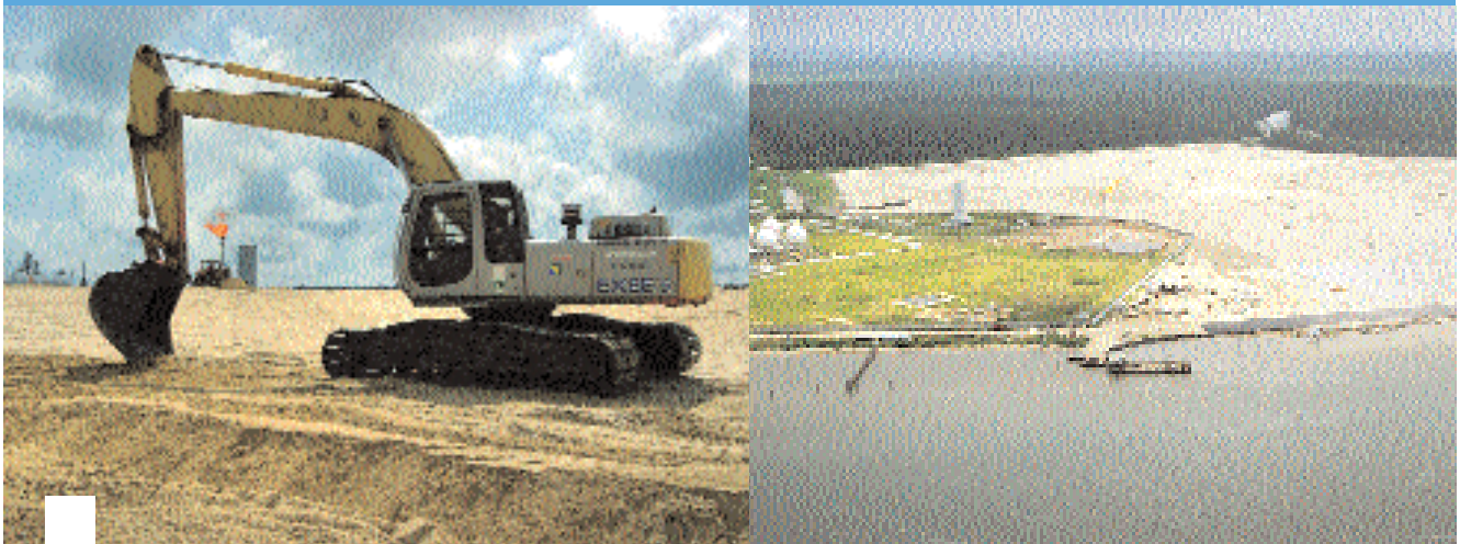
Construction on the gas-to-liquids plant at Escravos on the Niger Delta in Nigeria commenced earlier during 2006.
