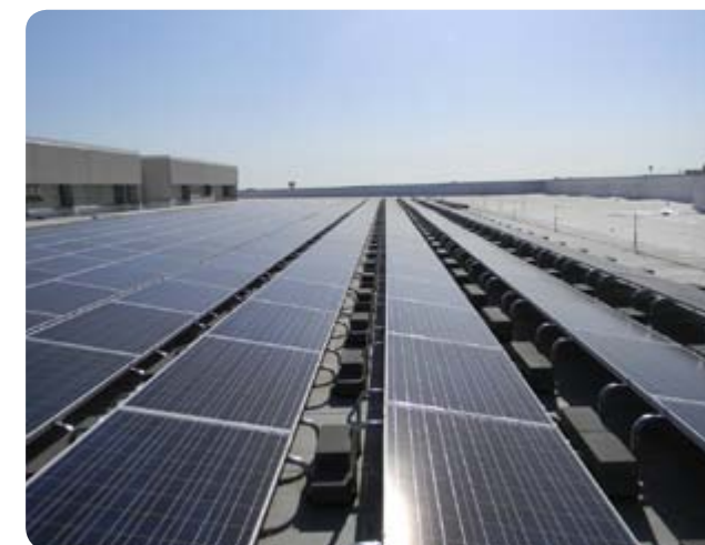
Cisco solar array at the Allen, Texas, data center
