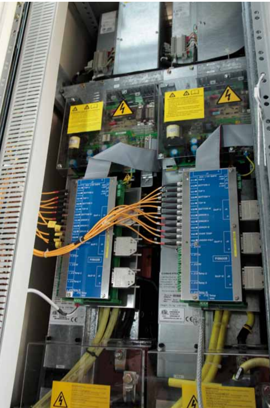
The Hesop system recovers tram braking energy and returns it to the grid.
