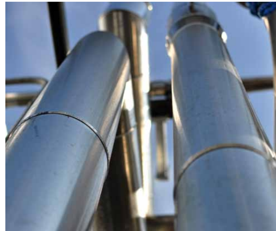
Detail of a carbon capture system installed by Alstom at the EDF power plant in Le Havre.
