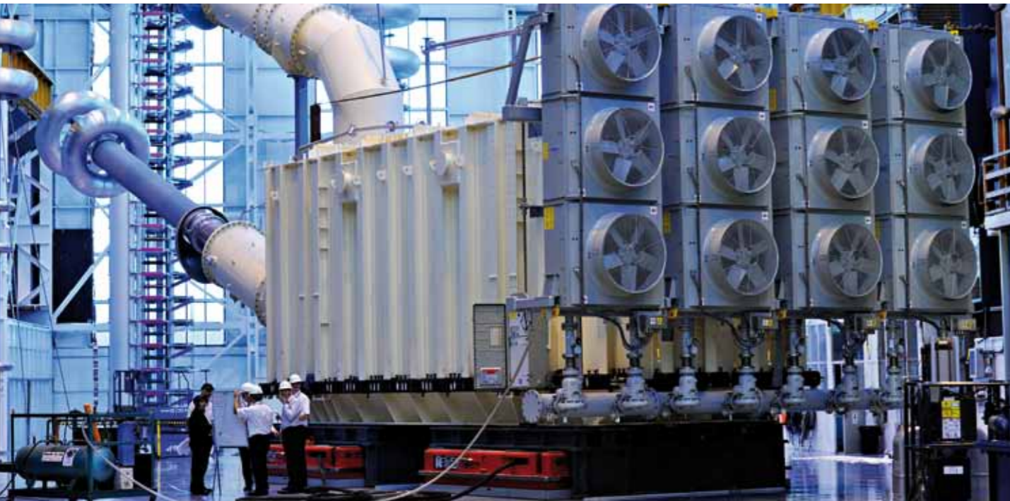
A UHVDC transformer for the Rio Madeira project.
