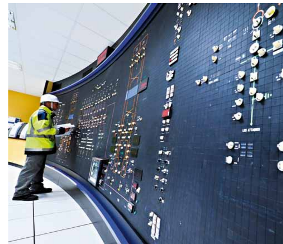
The control room for the IFA 2000 project linking France to the United Kingdom.
