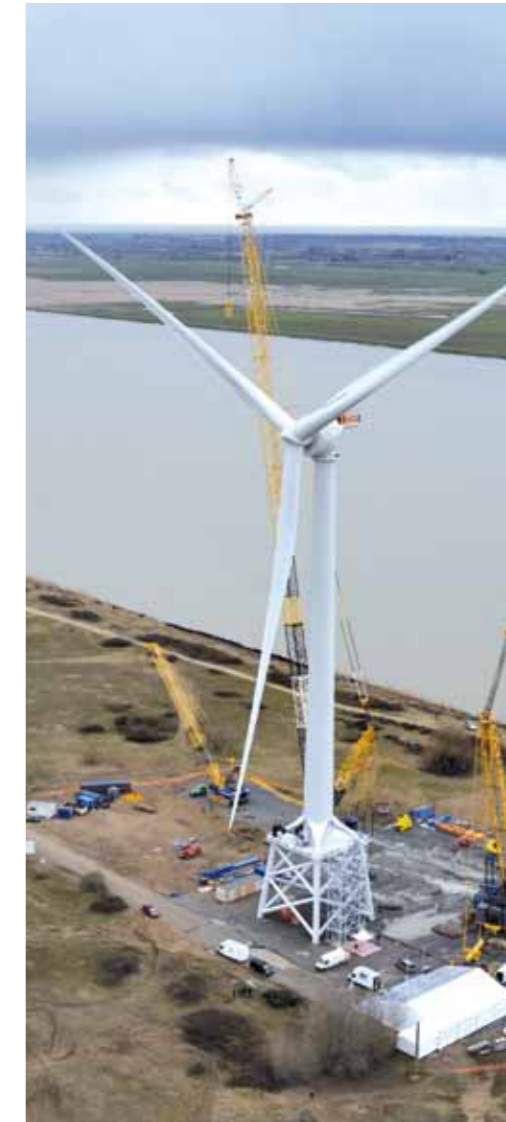
The first Haliade offshore wind turbine, at the Carnet site in France.
