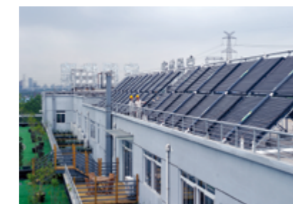
Rooftop solar water heaters of the logistic company of Baosteel Development
