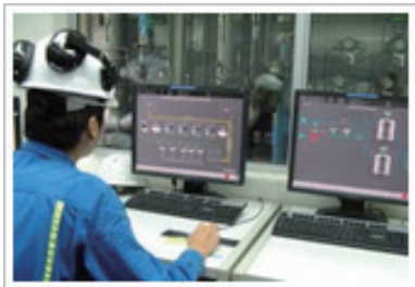
Main control room
