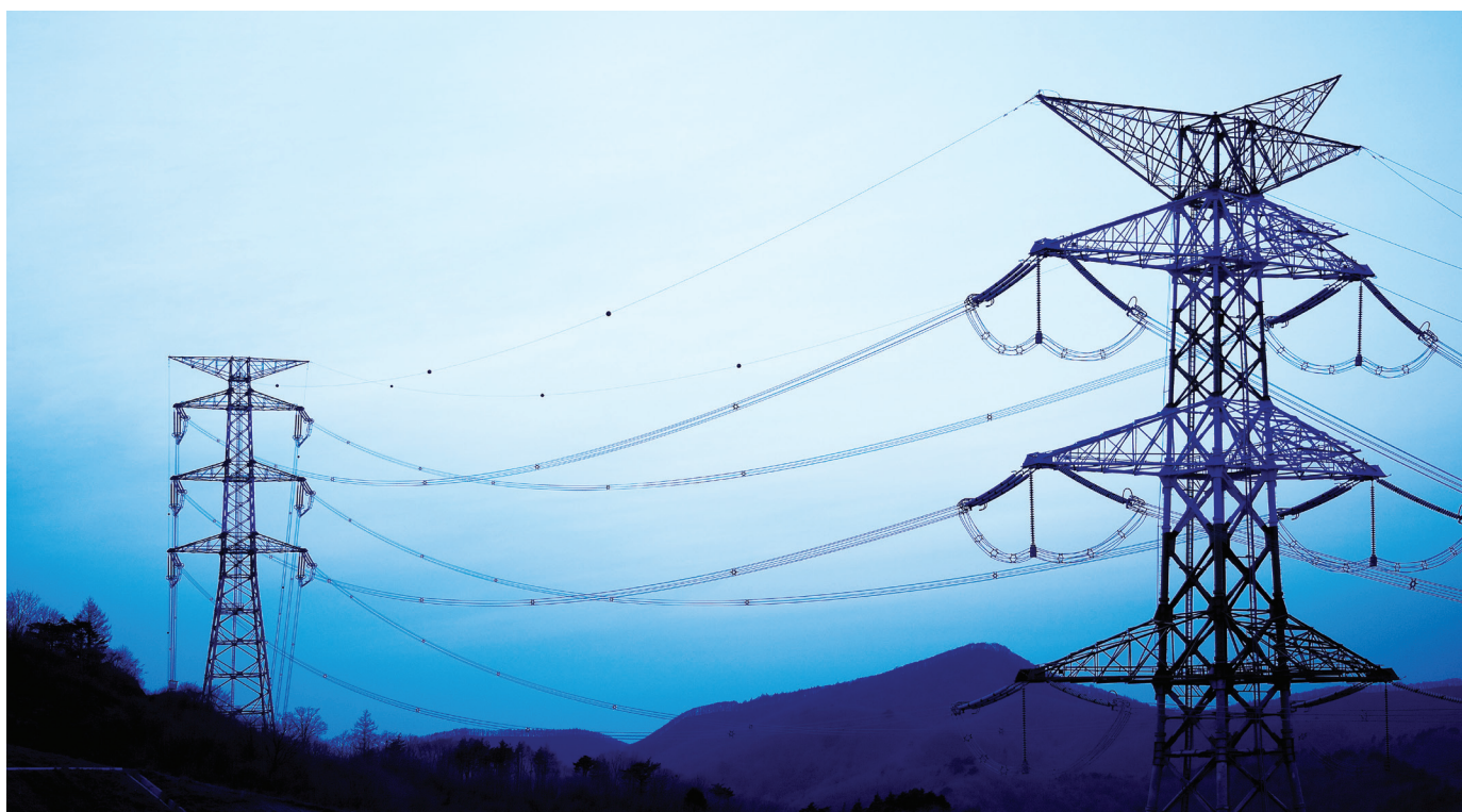
▶ SinTaebaek transmission tower
