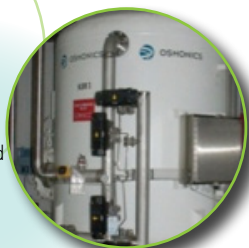
CCI Mersin Plant sand and activated carbon filter system
