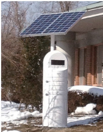
Monitoring post installed in Fukushima Prefecture
