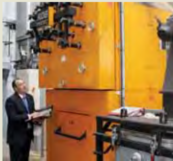
Replacing fuel oil with renewable woodchips as a source of energy is Gleneagles' first major step to carbon neutrality
