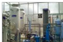
Biogas Purification Facility
