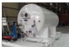
Liquefied Carbon Dioxide Storage Facility
