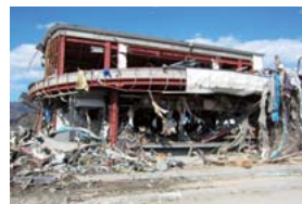
The tsunami devastated the Takata Branch, sweeping away the building front and ATMs.
