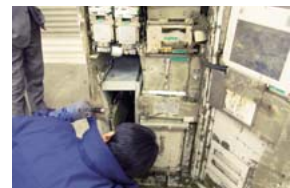
The tsunami caused major damage to 20 ATMs. Engineers tackled tasks such as repairing ATMs with case damage.
