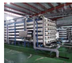
Hitachi Plant Technologies' Reverse osmosis desalination system
