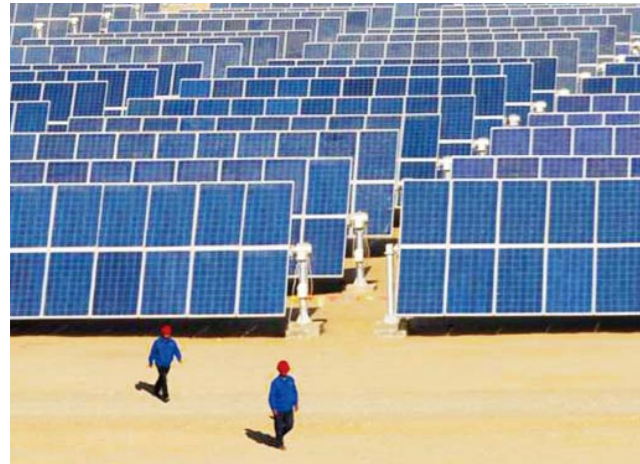
光伏电站 Photovoltaic power station
