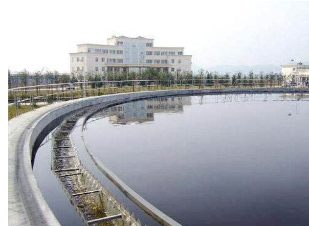
宜昌临江溪污水处理厂 Linjiangxi Sewage Plant at Yichang, Hubei Province
