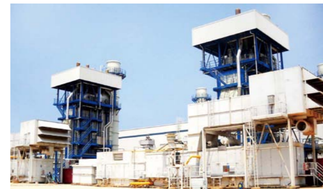
电厂的动力岛（燃机组）外景 Exterior of the power island (generator units)
