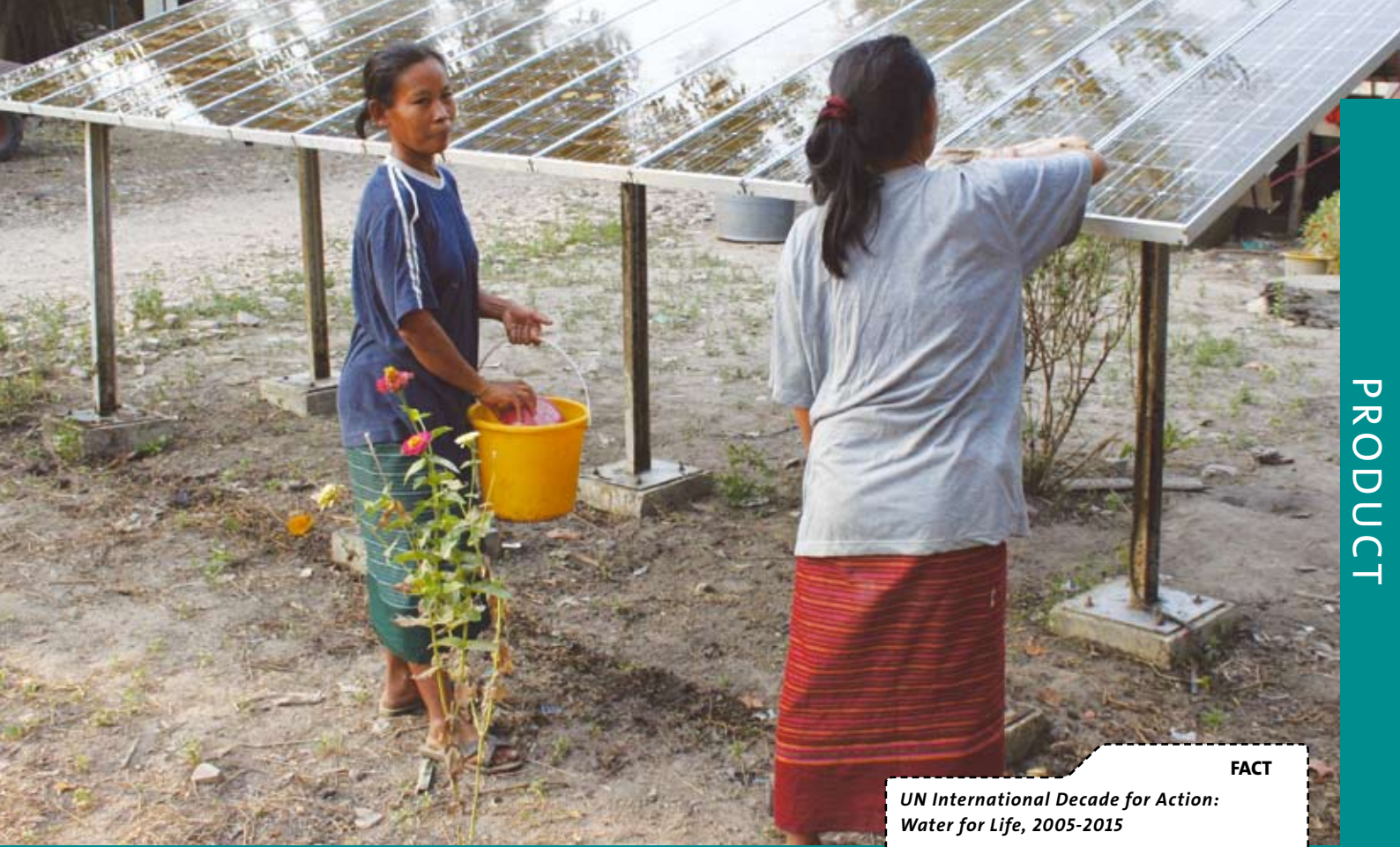
Women in Kudchalert Village cleaning the solar panels used for the SQFlex system.
