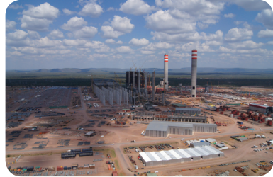
The new Medupi power station in Lephalale, Limpopo province
