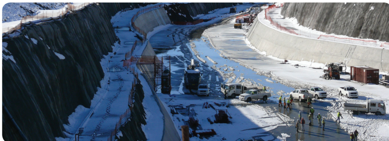
Snow covers the intake canal of the Ingula pumped storage scheme under construction near Ladysmith
