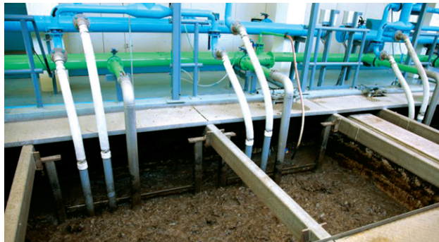
Waste water recycling plant, Mysore campus
