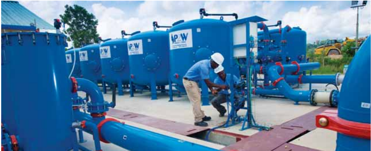
A new water treatment plant is in place at Iduapriem, in Ghana. It uses reverse osmosis to convert used process water from the plant into safe water which is discharged back into the river system near the mine. The process primarily removes the arsenic from the water
