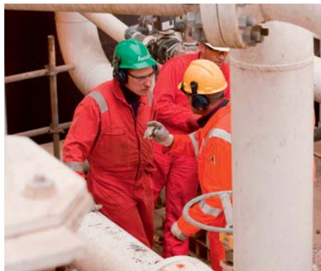
Maintenance personnel onboard the Chirag platform in Azerbaijan
