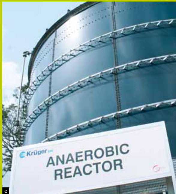
c The new effluent treatment plant at our brewery in Kumasi, Ghana removes organic matter from wastewater that previously flowed to a river.
