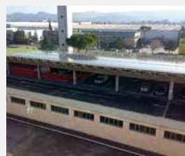
A 198 kWp photovoltaic plant on the roof of the car park at the Banca Popolare di Ancona Esagono Management Centre at Jesi.
