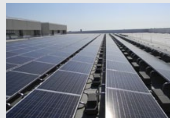
Cisco solar array at Allen, Texas data center.
