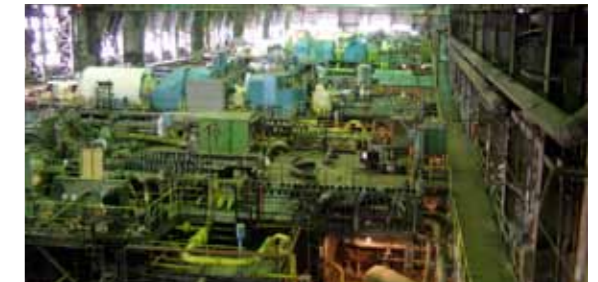
ACHINSK ALUMINA REFINERY, TURBINE AREA
