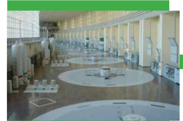
TURBINE ROOM OF SAYANO-SHUSHENSKAYA HPP
