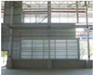
Ventilation through large louvers on the outside wall
