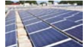
Solar power generation system on the roof of SMCA
