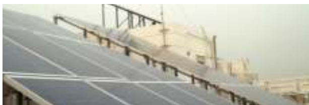
11.34 kWp Solar System installed at Mahindra Chloris
