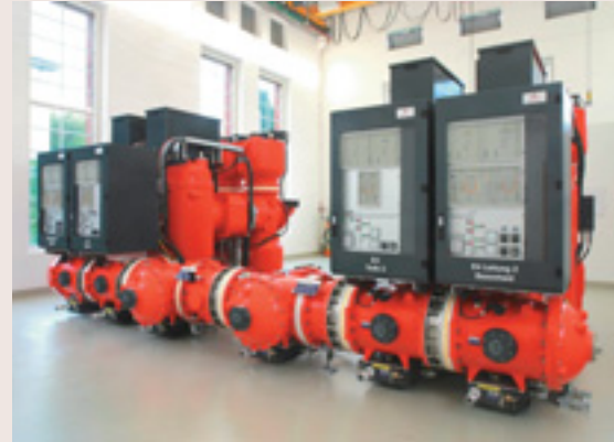
F35, AN ECO-DESIGNED SUBSTATION.
