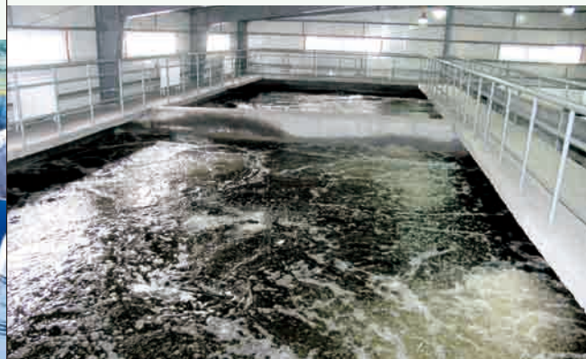
◆ Treatment pool for the recycled water of Wuhai Thermal Power Plant
