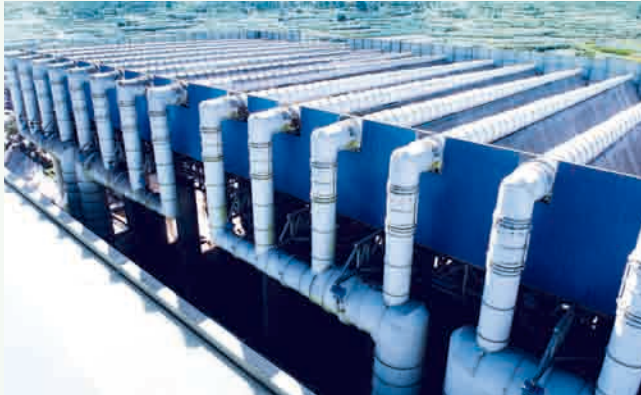
◆ Air-cooling island of Phase 3 of Huaneng Shang'an Power Plant
