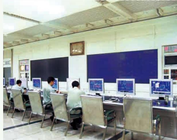
◆ Central control room
