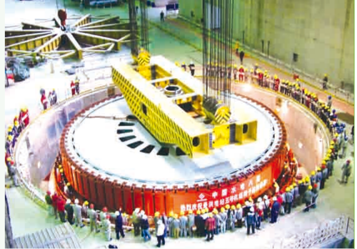
◆ Installing the rotor of the first hydro turbine generating set in Jinghong Hydropower Station
