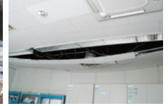
A collapsed ceiling at the Shirakawa Plant
