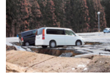
Quake soil liquefaction damage in the parking lot at the Shirakawa Plant
