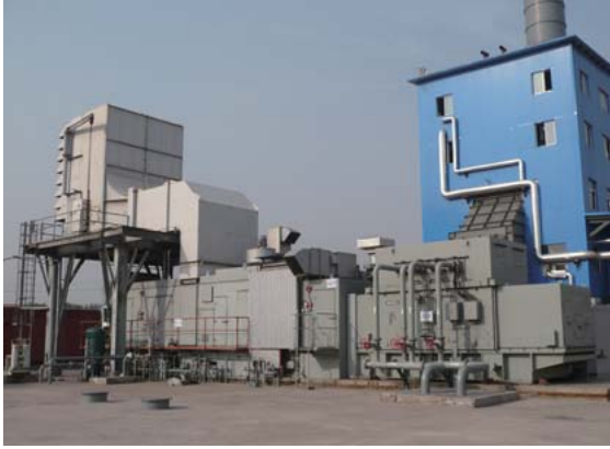
Cogeneration power plant equipment: Jingyuan Redian in China adopting the H-25 gas turbine
