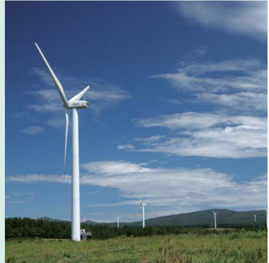
Rokkashomura-Futamata Wind Power Station
