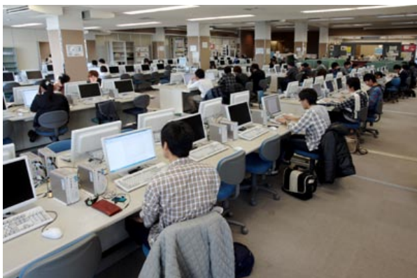
180 thin client terminals installed in an open space for IT education terminals
