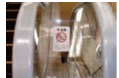
Safety Measures for Escalators
