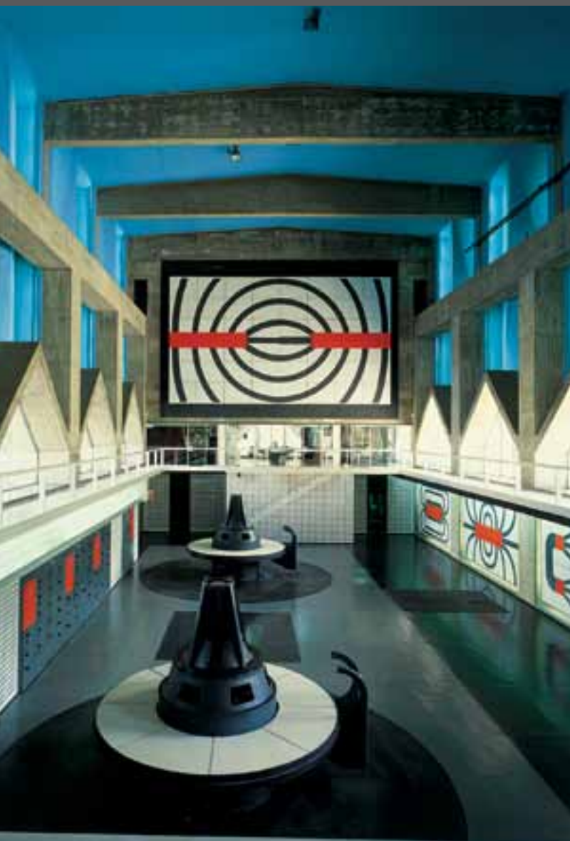
Proaza Hydroelectric Power Plant
