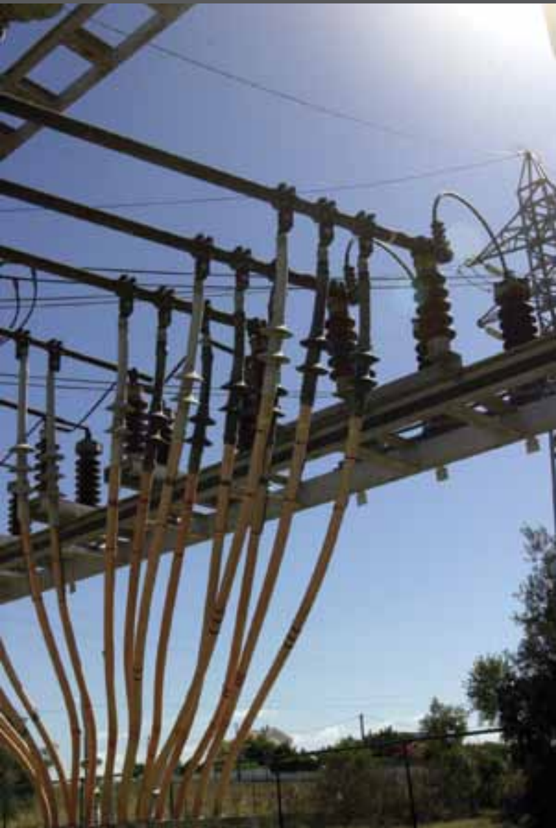
S. Francisco Substation
